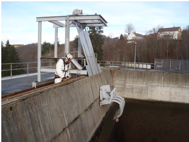
Figure 2.4: Wire rope trash rack cleaner at Leirfossen
