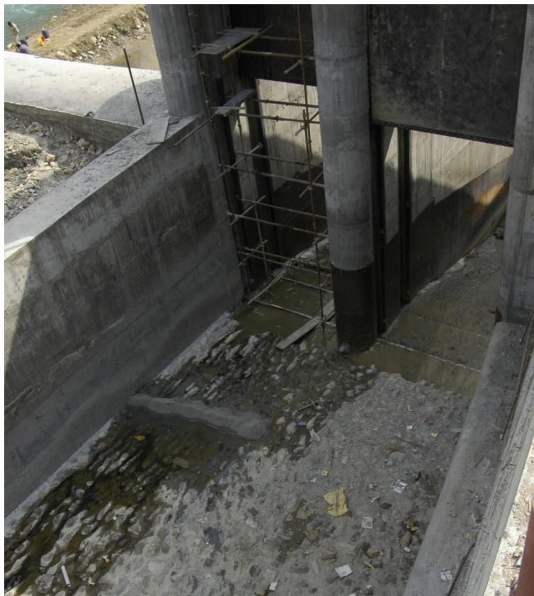
Figure 3.11: Undersluice flushing gates at Lower Modi I, Nepal
