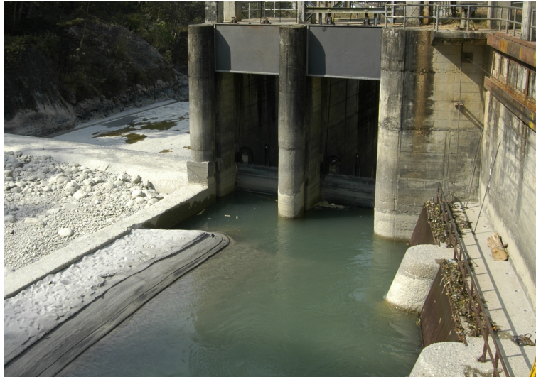
Figure 3.18: Downstream flushing gates at Modi Khola HEP
