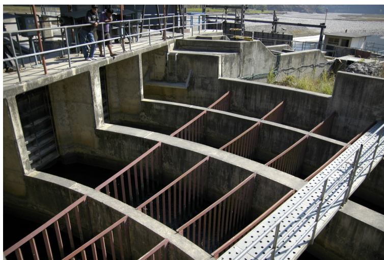
Figure 3.6: Flow tranquilizers at Jhimruk Hydropower Plant
