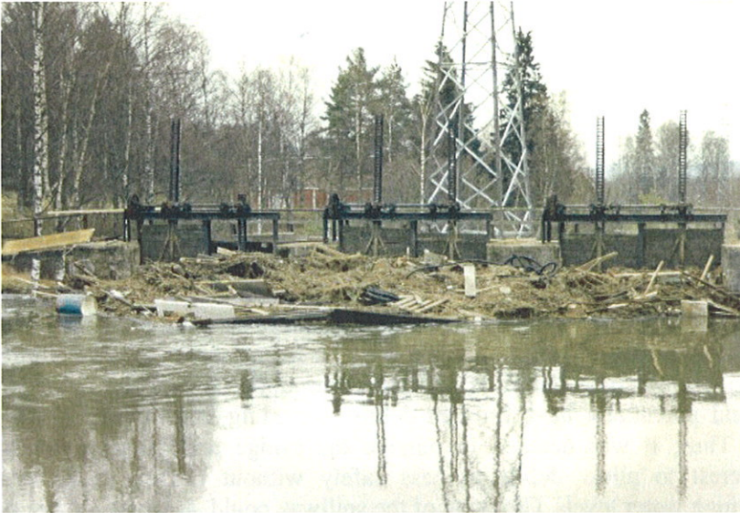
Figure 5.13 Debris at small intake dam, 1987 (photo: V.N.Svendsen)
