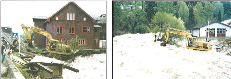
Figure 5.19 Attempts to protect Fonstad (left) and Moksa power plant (right) on 1 June 1995 (photo: MGE)
