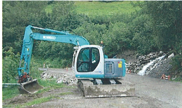
Figure D-11 Repair work on the main road from Vinstra to Skåbu (Olstappen) after erosion damage from flood in a small tributary to Vinstra River, August 2000
