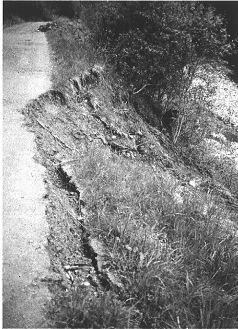
Figure B-8 Slides between the road and the reservoir at Vinkelfallet
