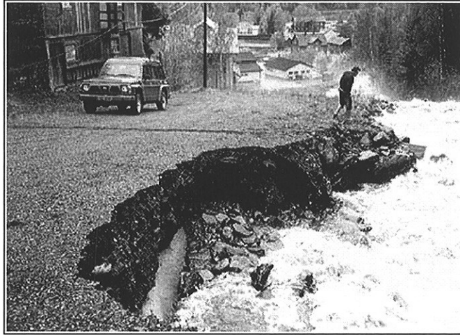
Figure B-1 The mechanical engineer inspecting the river banks close to Moksa 1 (the old power plant) on 1 June 1995 – notice erosion around the pipeline (photo: MGE)
