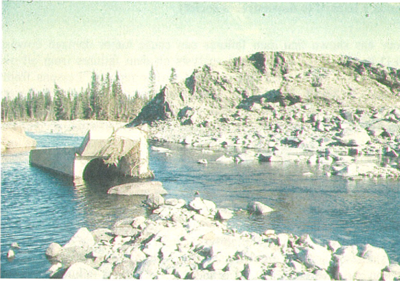
Figure 1.2 Roppa Dam after failure (photo: Department of Hydraulic and Environmental Engineering, NTNU)
