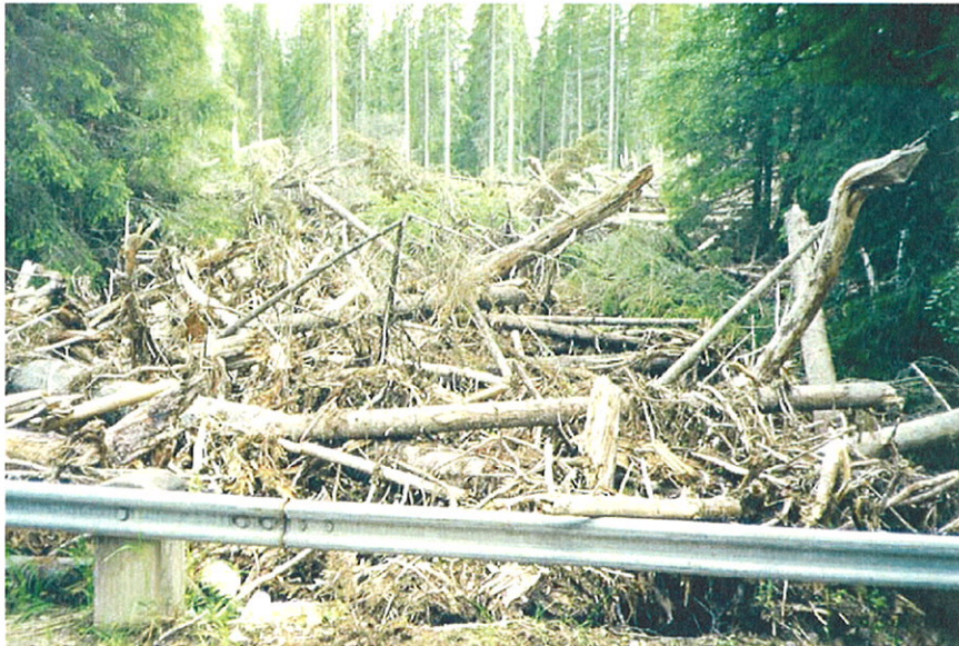
Figure C-4 Looking upstream from the Stora Göljån culvert. Accumulated debris in the old river course
