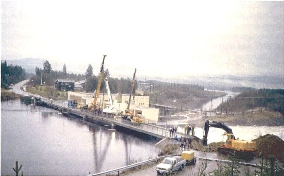
Figure 5.10 Preparations for blasting of western embankment during the 1986 flood at Lutufallet (photo: O.J.Olberg)
