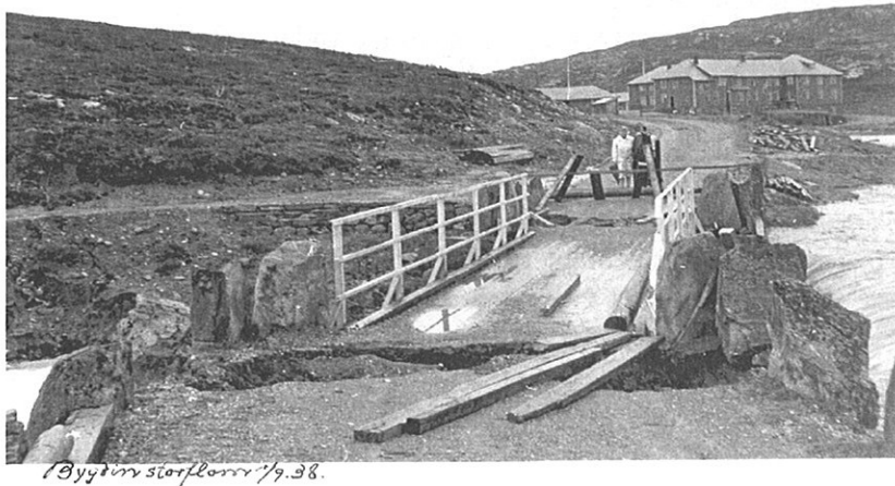
Figure 5.8 Damage to southern road bridge downstream of Bygdin (photo: GLB)
