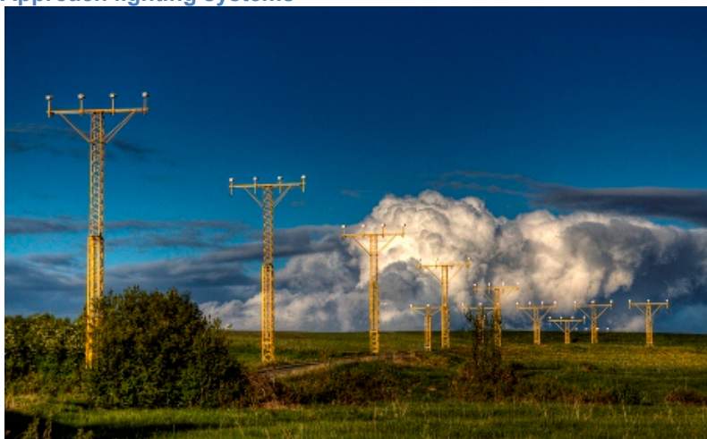
Figure 1; Approach lighting structures (Frangible Composites)
