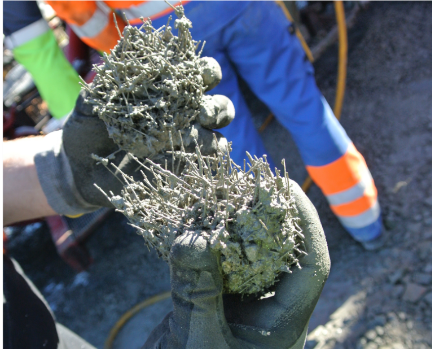
FIGURE 5.2: During casting of the polymer fiber mix, a plug formed in the pump.
