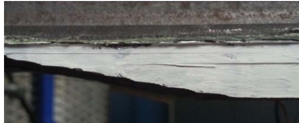
Figure 48 – Delamination started at the tapering on beam #48
