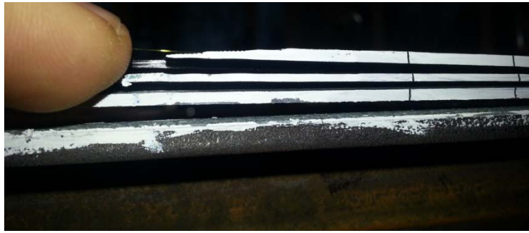
Figure 55 – Delamination in different layers, beam #23
