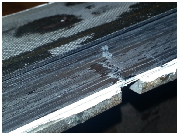
Figure 59 – Fiber rupture, beam #24
