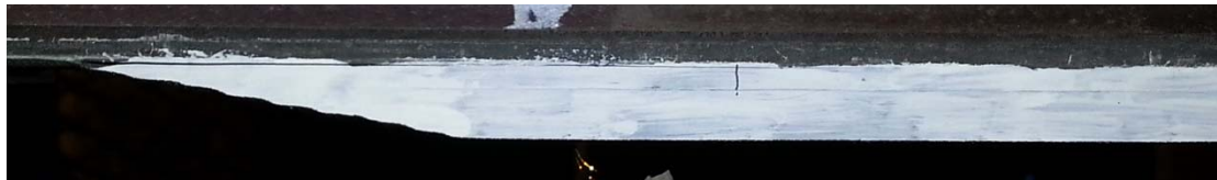
Figure 50 – Delamination from the left side of beam #49
