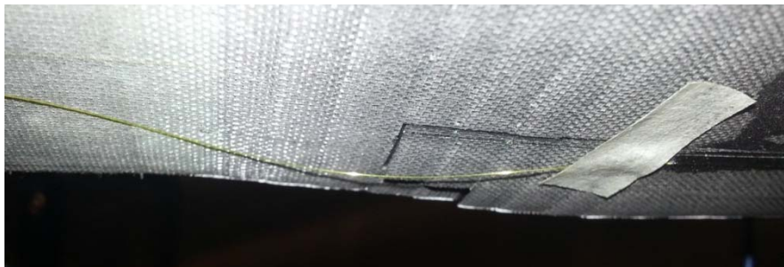
Figure 54 – Part of the patch delaminated on beam #23
