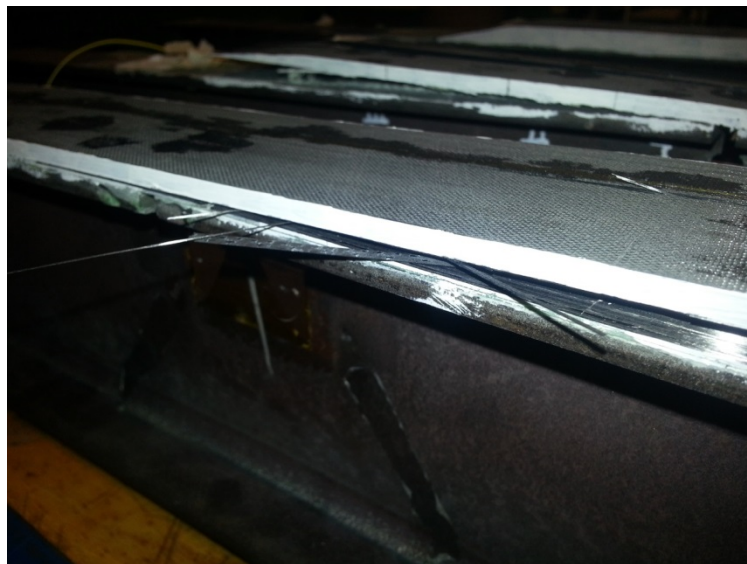
Figure 57 – Shredded fibers from inside the laminate, beam #23
