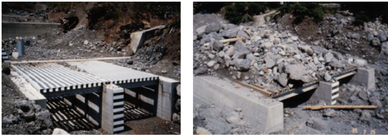
Figure 3.2: A 20 meter long and 10 meter wide debris flow breaker in Mount Yakedake, Japan. The left picture is before a debris flow has occurred while the picture on the right is after stopping the debris flow (Mizuyama, 2008)
