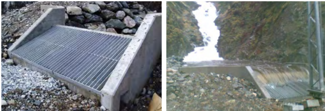
Figure 3.6: Self cleaning grids in Langhelle. On the right is the self cleaning grid during a flooding (Photo: John Endre Fossmark) and the left when there is normal flow (Photo: Jeanette Gundersen).
