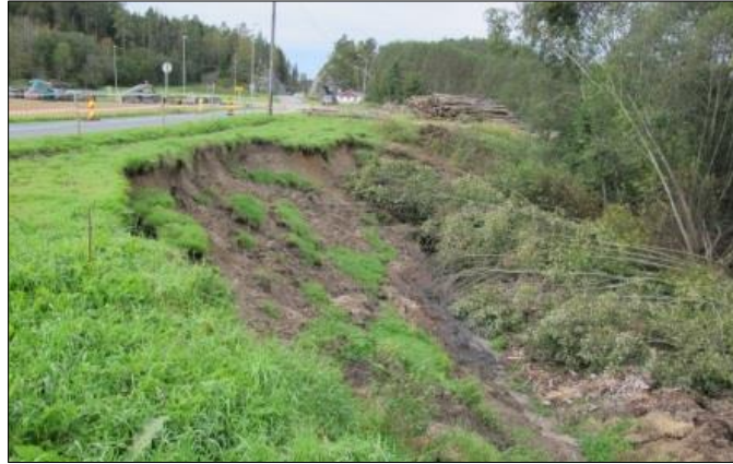
Figure 2-2 Soil slip caused by a weak layer, Åby in Telemark County, Norway (Håland, 2012)
