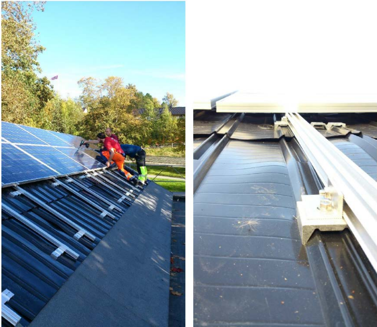
Fig. 1.13. Left: The installation of the PV modules on the InterSole system. The HDPE membrane is visible on the middle part of the roof. Right: A close-up of the aluminium profiles and the membrane (Good 2015).
