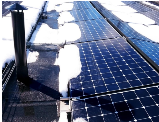
Figure 2.8: Cast shadow from the vent pipe at Block 5, 12:40 March 8th. (Photo by L. Ødegården)
