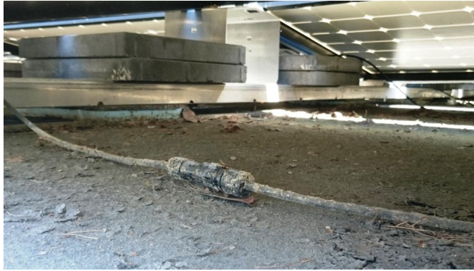
Figure 2.4: One of the MC4 connection cables lying on the ground, covered in dirt. (Photo: L. Ødegården)
