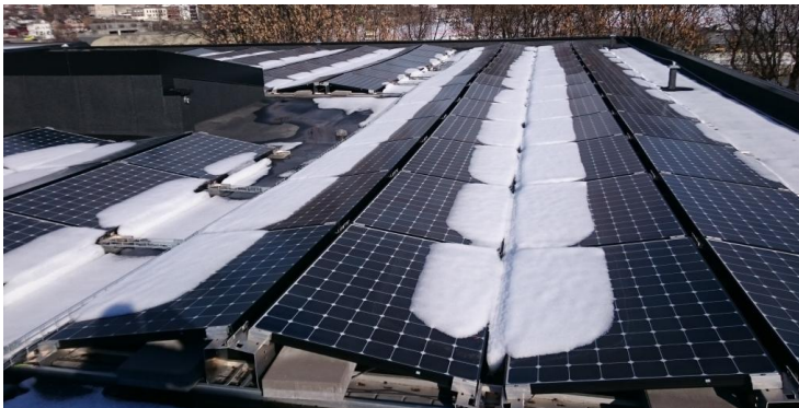
Figure 2.3: A photo of a part of the roof of Block 4 from March 10th, while there was still snow on the modules. (Photo: L. Ødegården)
