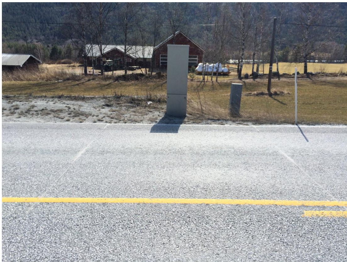
Figure 13: Picture of WIM 540109. Two cables and one processing unit box, the big box in the middle of the picture, can be seen. Photo: Torbjørn Haugen.
