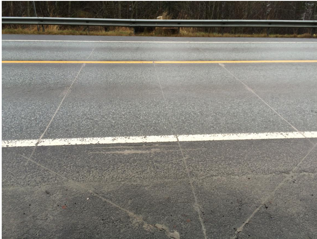
Figure 9: Picture of WIM 1740104. The location of the cables can clearly be seen. Photo: Torbjørn Haugen.
