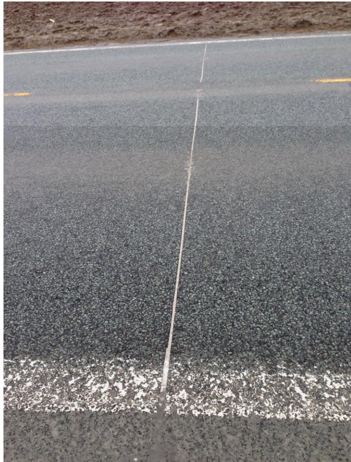
Figure 4: Strip sensors (piezoelectric) mounted in the asphalt. Photo: Torbjørn Haugen
