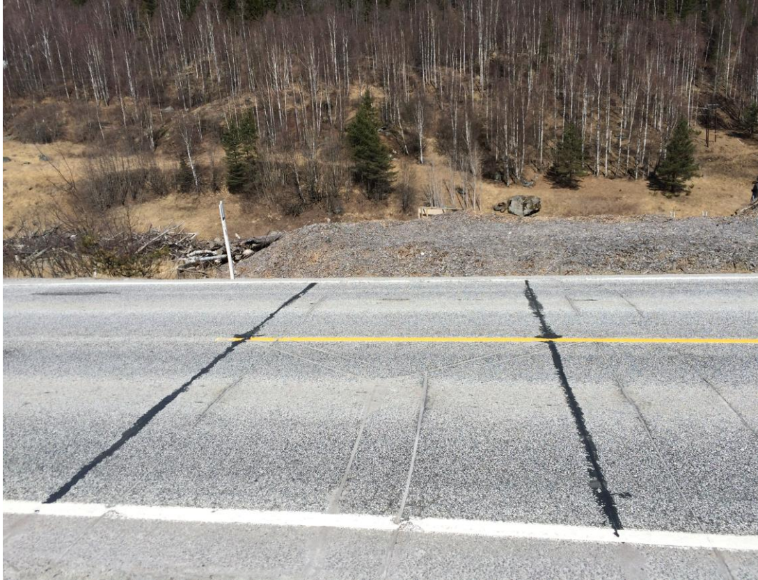
Figure 12: Picture of WIM 540031. Cables at the southbound WIM site. The thick black lines are due to some surface filling. The pothole cannot be seen in this picture. Photo: Torbjørn Haugen.
