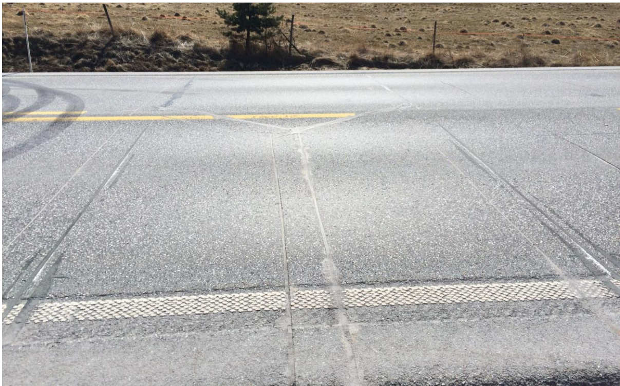
Figure 11: Picture of WIM 540032. The piezoelectric cables of the northbound WIM site can be seen. Photo: Torbjørn Haugen.
