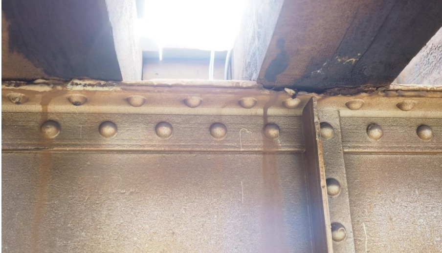
Figure 30, damage in top flange of crossbeams. Photo: Gunnstein Frøseth
