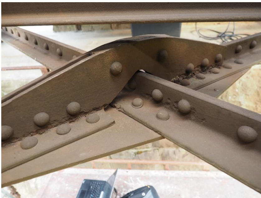
Figure 29, damage in connection of bottom bracing. Photo: Gunnstein Frøseth
