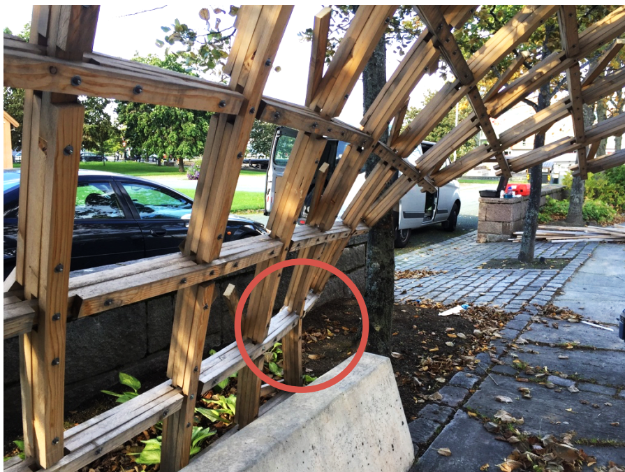
Figure 2.17: The outmost lath of the support failed in bending under asymmetrical loading
