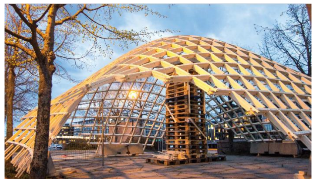
Figure 4: The lifting tower during erection. Credits: Steinar Hillersøy Dyvik and John Haddal Mork
