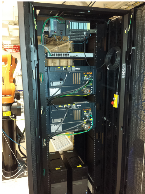
Figure A.1: The installed control cabinet for the Agilus robot cell
