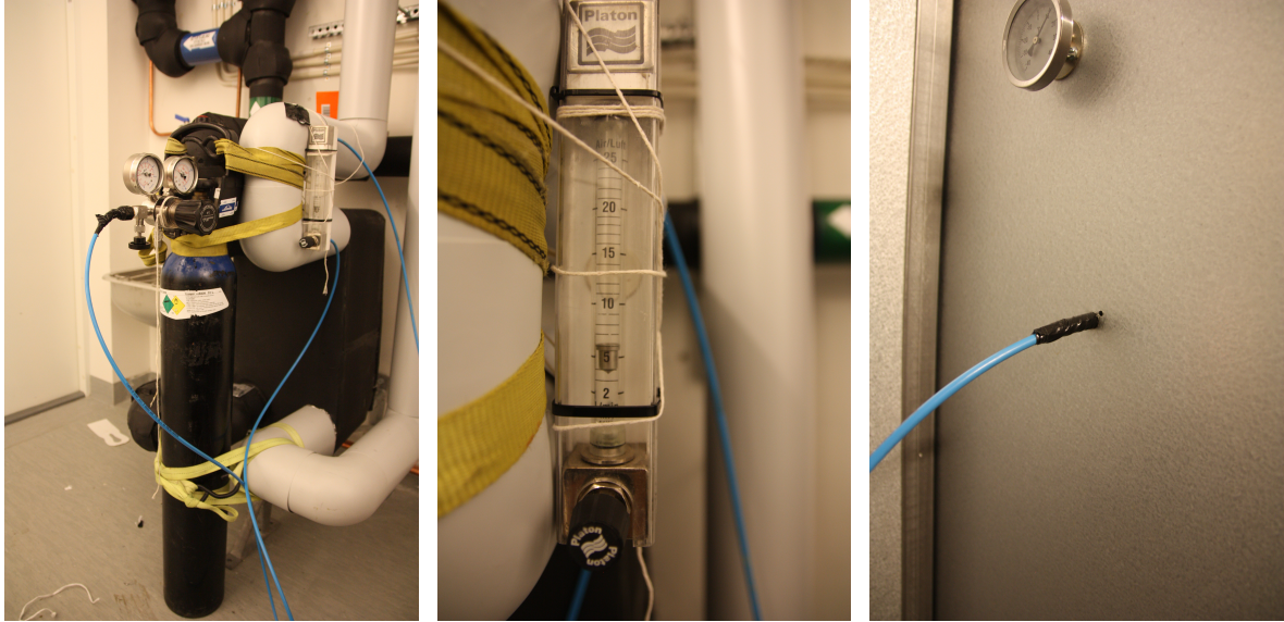
(a) The cylinder is tightly secured to prevent it from falling over. (b) A rotameter is used to ensure right gas dosage (c) The gas is injected directly into the air handling unit to ensure proper mixing
