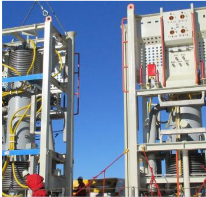
Figure 5.7 Two 5MW contra rotating subsea multiphase compressors for the Gullfaks subsea wet gas compression.
