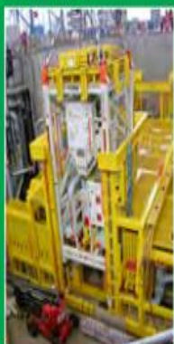
Fig. 1: Installation of the OneSubsea Pump Module into Pump Station during SIT for the Exxon Julia project
