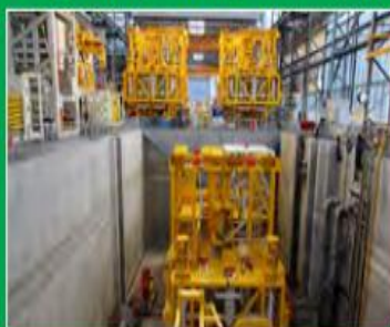
Fig. 10: Jack & St Malo Pump Stations in the Factory Pit for System Integration Test (SIT)
