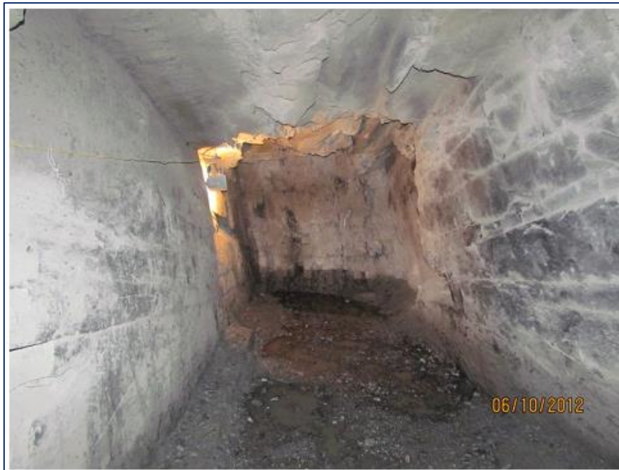
Figure 3-7. Rock face at RD 114.0m in power house drift (PH-1) Alternative IV
