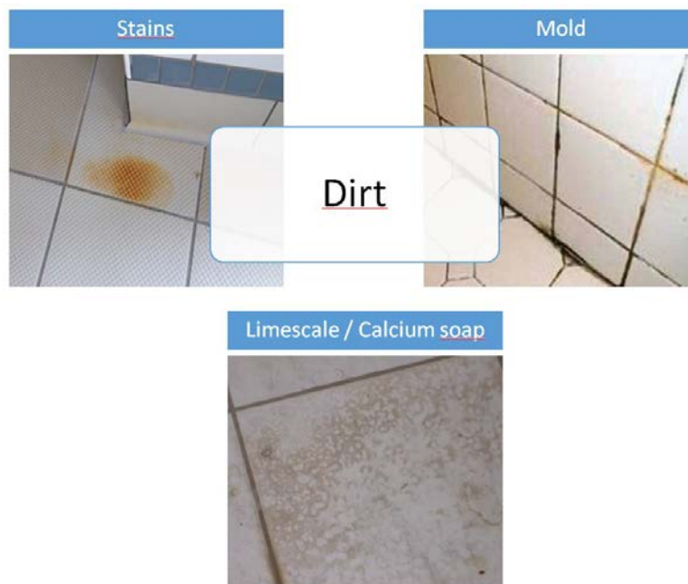
Figure 4-4: Dirt; stains (Sys teco, n.d), mold (Jaka, 2015), limescale/calcium soap (Knoji, 2013)
