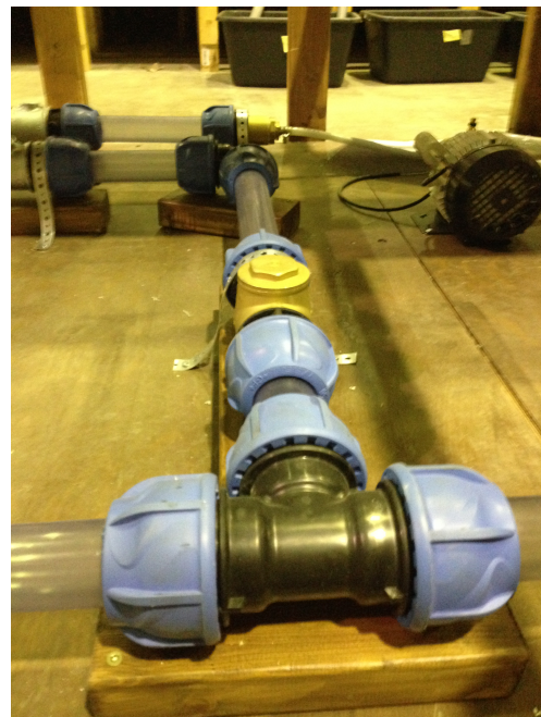
Figure 3.34: Pipe connections with one-way valve located on the big frame.
