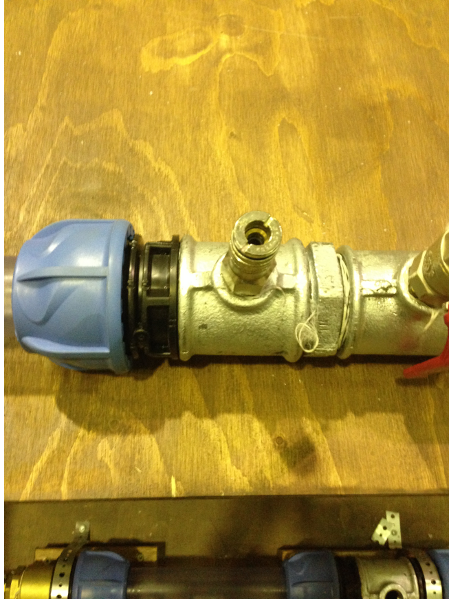
Figure 5.5: The compressed air connection point in the system.
