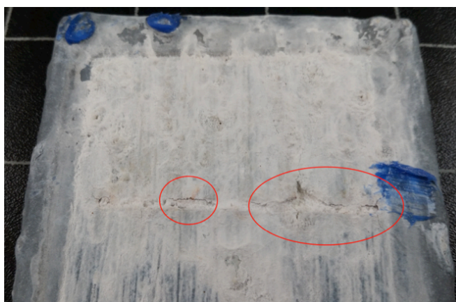
Figure 4.2: Blistering and cracking of the topcoat near the scribe on the Zn epoxy DFT 150 \mu\text{m} . The picture is taken after 20 cycles of exposure.
