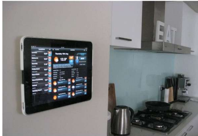
Figure 6.10: A wall mounted tablet 1
