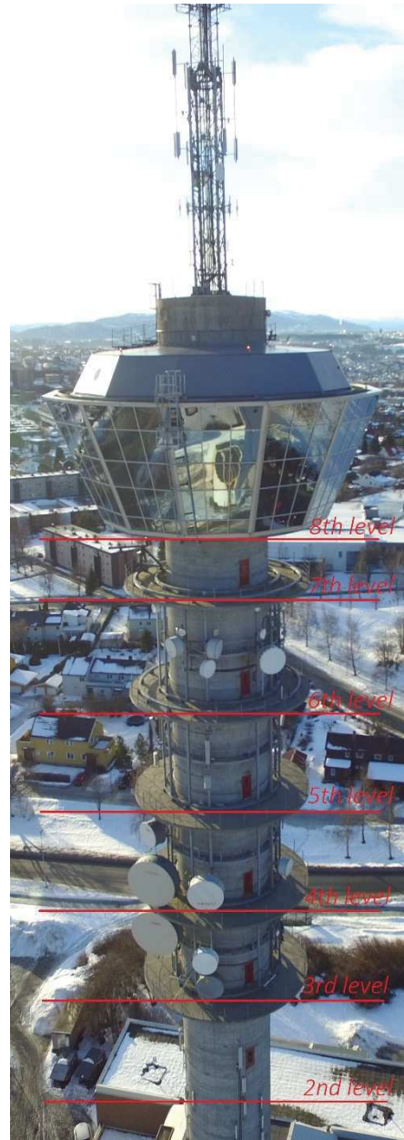
Figure 10 - Selected, observed levels on the tower from the angular method. Levels from 3 to 8 are located right under the standings and main gallery.
