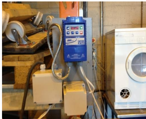
Figure 4.4a: The pump/flow regulator, while in use
