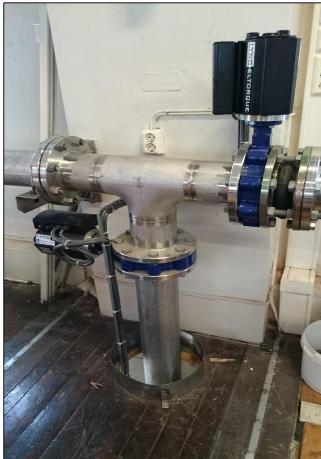
Figure 18: Tee junction in the Pelton-loop. The pipe on the left hand side is connected to the pump at ground level, while the pipe to the right is connected to the nozzle on the Pelton turbine. The vertical pipe leads down to the weighing tank; this is only in use when calibrating. The pipes in the tee junction have a diameter of 100 mm.
