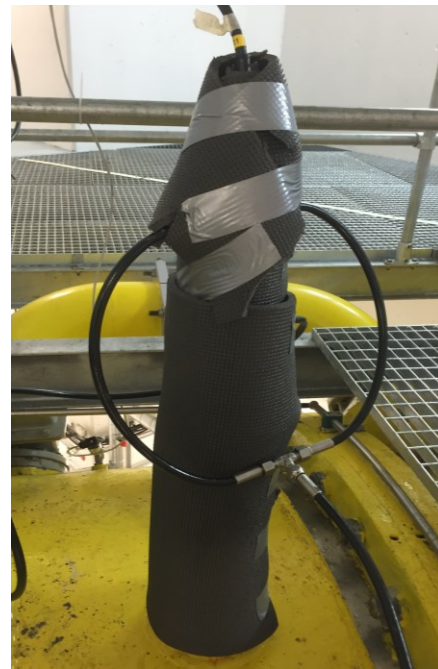
Figure 23 - Temperature sensor at inlet
