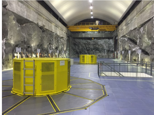
Figure 1 - Machine hall Leirfossene
