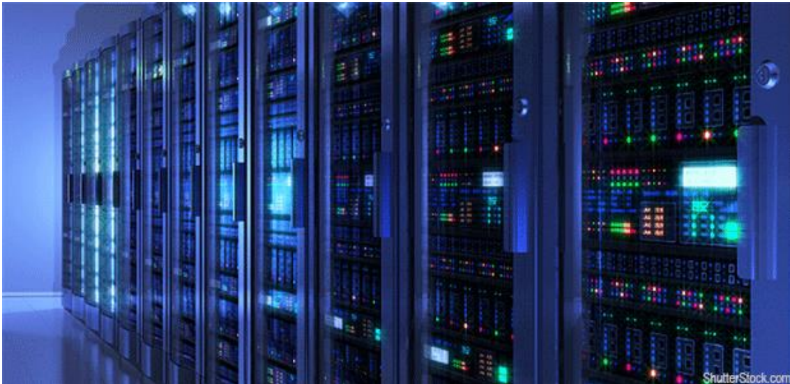
Figure 1. Example of servers in a data center [8]
