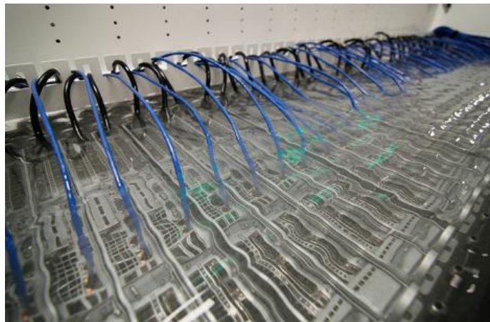
Figure 5. Immersion liquid cooling in data centers [18]
