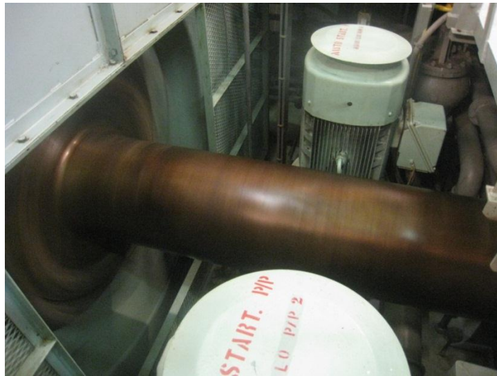
FIGURE 18: MAIN ENGINE LUBE OIL PUMPS, VESSEL X1-1
