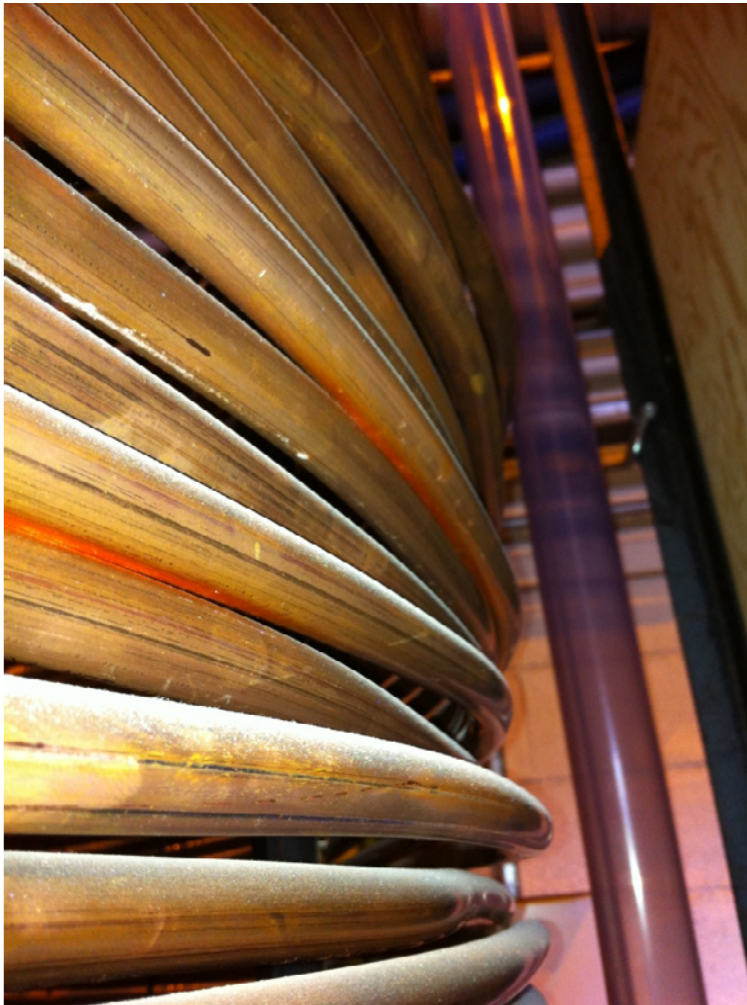
Picture 6.1; non-uniform copper pipe circumference.
