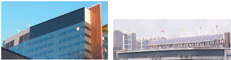
Fig. 1. The SolarWall PV/T facade at Concordia University, Montreal (left), and the SolarWall PV/T installation on the Olympic village in Beijing (right). SolarWall® PV/T system, photos courtesy of Conserval Engineering.
