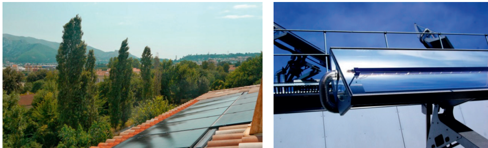
Fig. 2. A roof integrated PV/T system in Marseille, southern France (left, photo courtesy of DualSun), and the Absolicon PV/T installation to the local hospital in Härnösand (right, photo courtesy of Absolicon).
