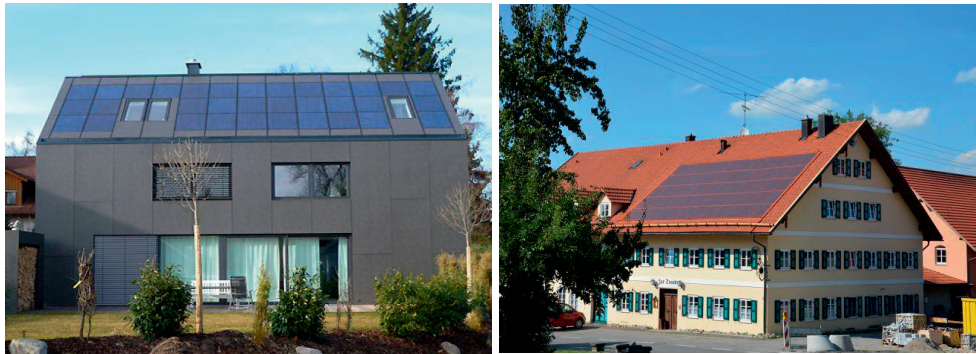
Figure 24. A building integrated PV/T system with Wiosun modules (right) and red PV/T modules by Wiosun. Photo: Wiosun [147]
