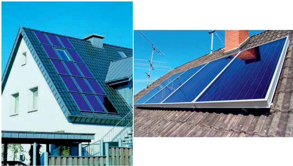
Figure 7. A building integrated (left) and a building added (right) solar thermal system. Photos © European Solar Thermal Industry Federation (ESTIF).
