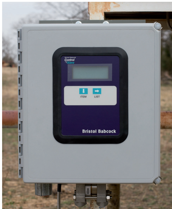
Fig. 1.11 – The RTU installed at the Noblin #2.
