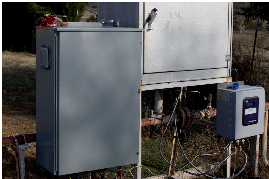
Fig. 1.22 – The Noblin #2 metering station. From left: network equipment box, chart meter cabinet, and RTU. The chart meter is no longer used, because gas rates are now measured by the RTU.
