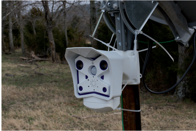
Fig. 1.19 – One of the two IP cameras installed on the Noblin #2. The cameras transmit live video feeds that can be viewed through the ROOKIE client application.
