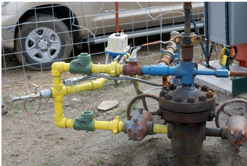
Fig. 1.9 – Noblin #2 wellhead. Pipes transporting gas are painted yellow, and pipes transporting water are painted blue.
