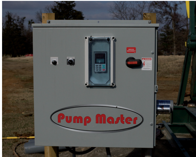
Fig. 1.18 – The pumping unit control box installed on the Noblin #2. The control box is connected to the RTU, and starts and stops the pumping unit.
