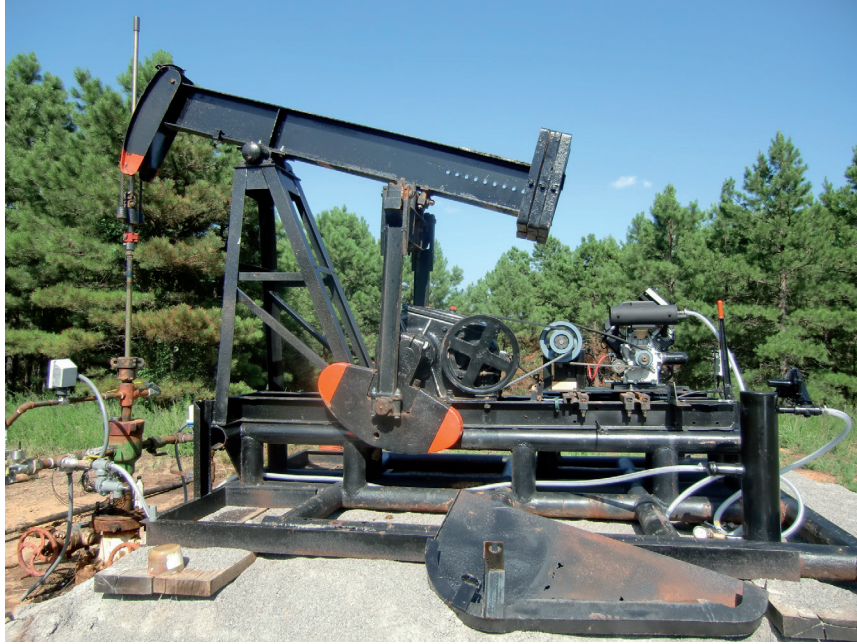
Fig. 2.31 – The pumping unit installed on the Anglin #3. Gas from the annulus is fed through a pressure regulator to the pumping unit motor.
