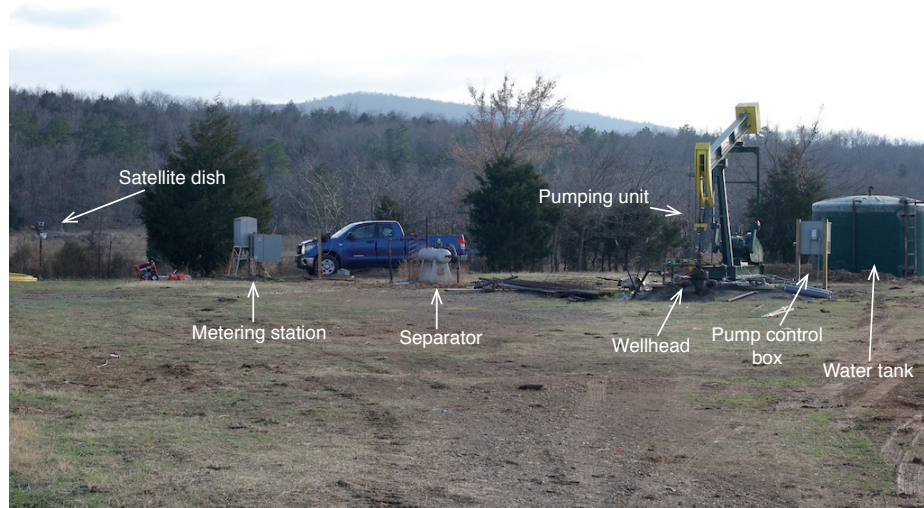
Fig. 1.7 – Noblin #2 wellsite. All major parts of the wellsite are marked on the figure.
