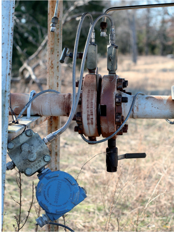
Fig. 1.2 – The pressure differential cell connected to the SPIDR unit to measure gas production rate.
