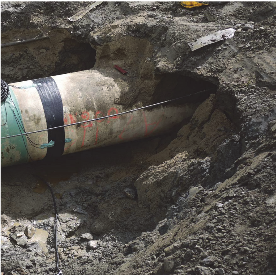
Figure 3.7: Excavated pipeline. The thin film sensors are beneath the black tape. The epoxy compound is there to keep the wiring in place during installation (Oosterkamp [45]). The thin film sensors at the left and right hands side failed in their function after a short time of operation.
