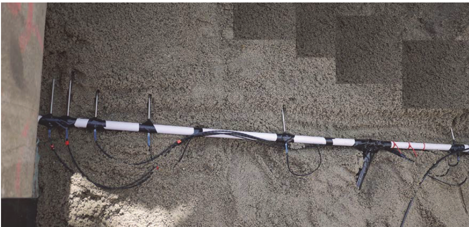
Figure 3.6: Sensor boom shown during its installation at right hand side of the pipe.
