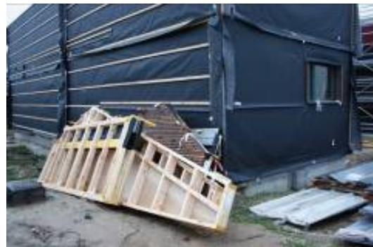
All components are assembled inside a factory. This industrialization should allow building without humidity. Unfortunately, the elements are stored outside in bad weather on the site.
