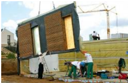
Most of the external timber cladding is put in place on site after the industrially produced components have been assembled.
