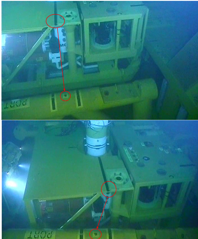
Figure 7.1: Alignment marks on Xmas tree and subsea structure
