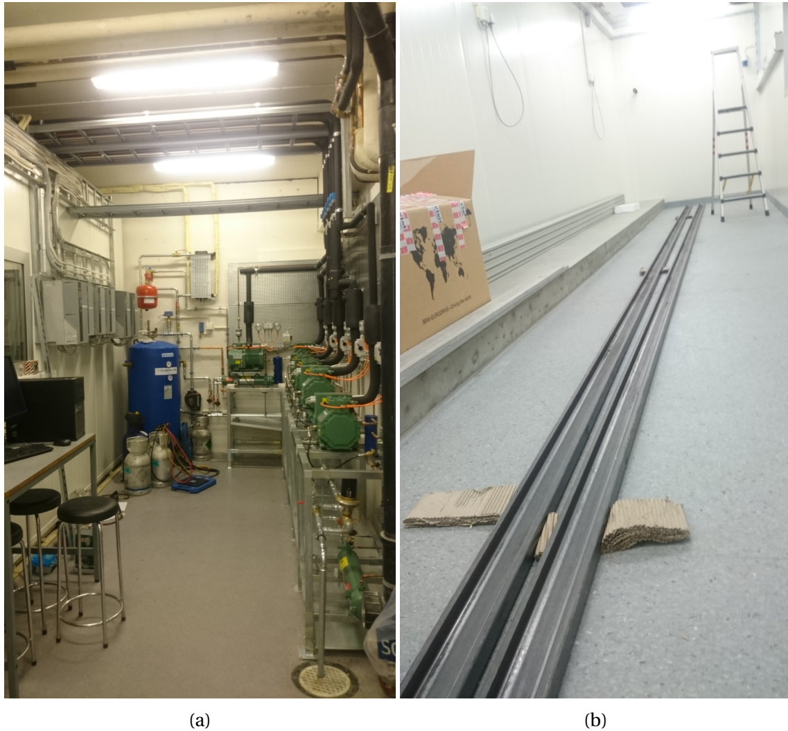
Figure 1.2: a) Snow lab control room b) Test track railings laying in the test room. Photos are shot on November 20th, 2015.
