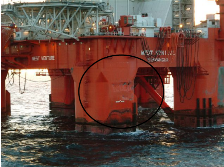
Figure 2.1: The semi submersible drilling rig "West Venture" after collision.
