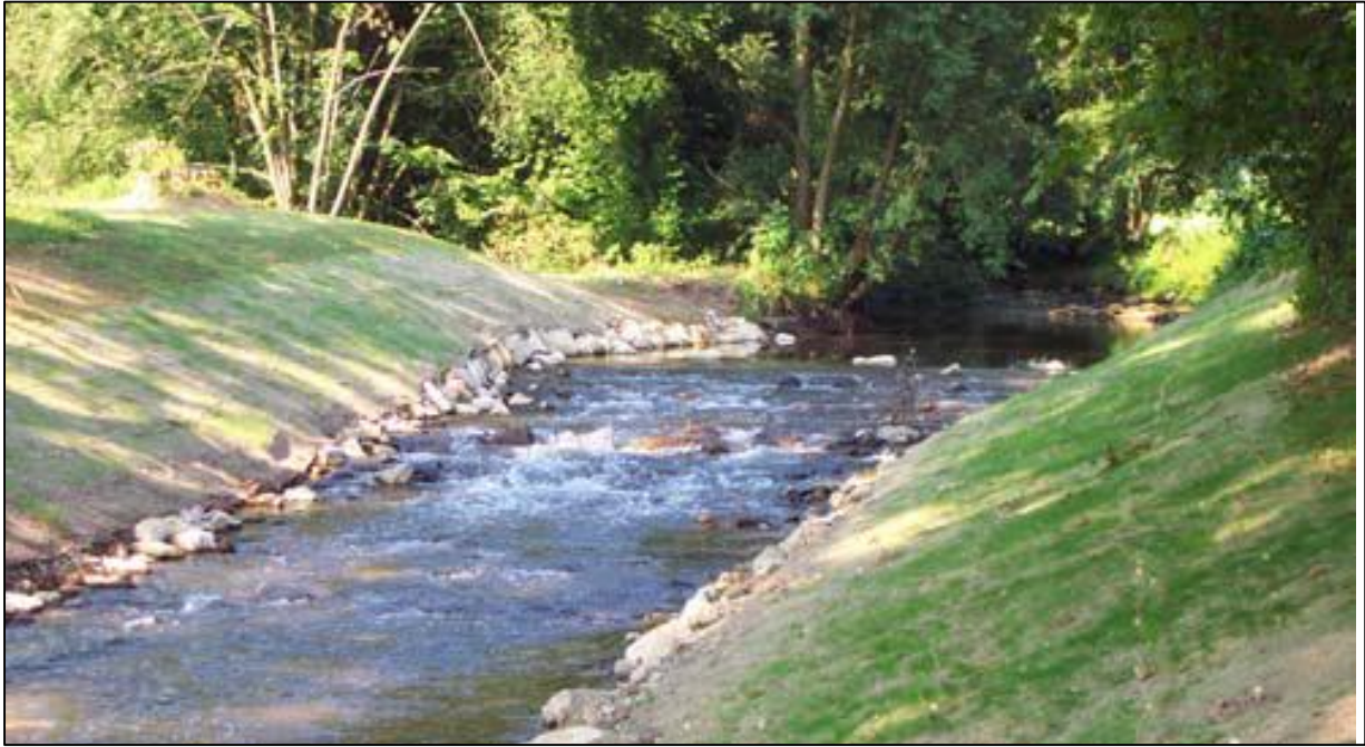
Figure 8. Rockfilled slide in the Aich River (LUBW, 2005)
