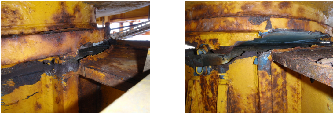
Figure 2.3: Crack in connections between leg and topside
