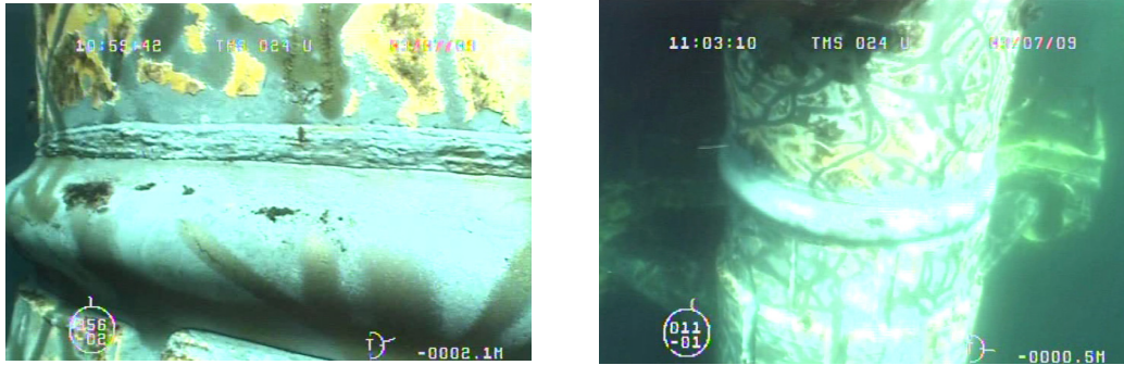
Figure 7.9: Buckling of splice joint at -2m
