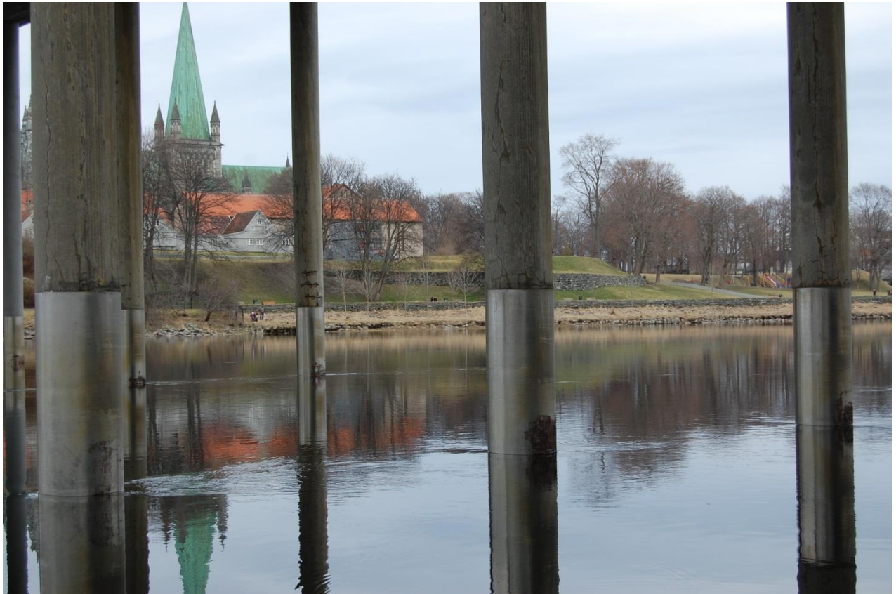
Figure 3.6 ASR in combination with corrosion of embedded reinforcement processes in zone 2-5. [fot. by Maciej Wisniewski & Krzysztof Wojslaw].
