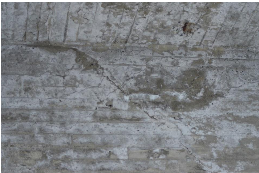
Figure 2.2. Map-cracking of a construction beam caused by ASR [ fot. by Maciej Wisniewski & Krzysztof Wojslaw].
