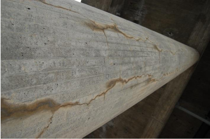
Figure 4. Corrosion of embedded reinforcement in column [ fot. by Maciej Wisniewski & Krzysztof Wojslaw].
