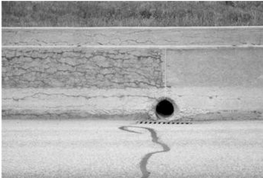
Figure 8.6 Barrier wall in Quebec-the section of the wall to the right of the picture has been treated with a silane sealer.
