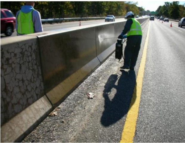
Figure 8.3 Photograph showing topical application of 40 percent-Silane Solution (solvent-based) to ASR-affected highway barrier.
