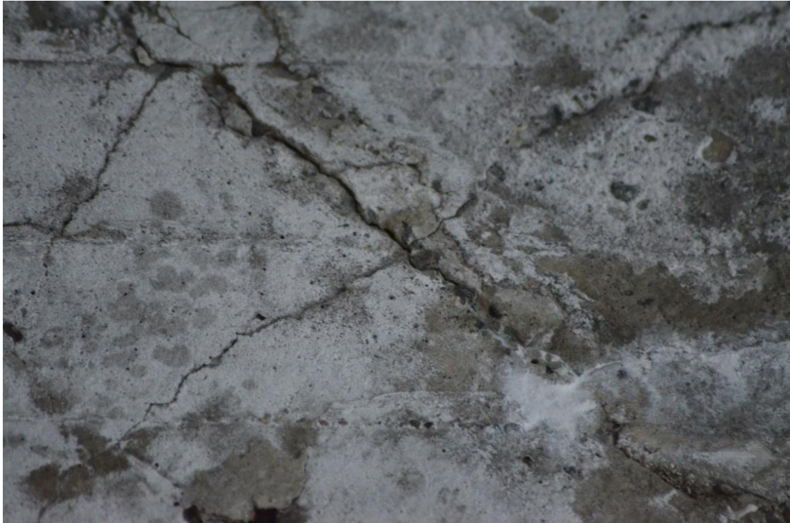
Figure 2.3. Map-cracking of a construction beam caused by ASR [ fot. by Maciej Wisniewski & Krzysztof Wojslaw].
