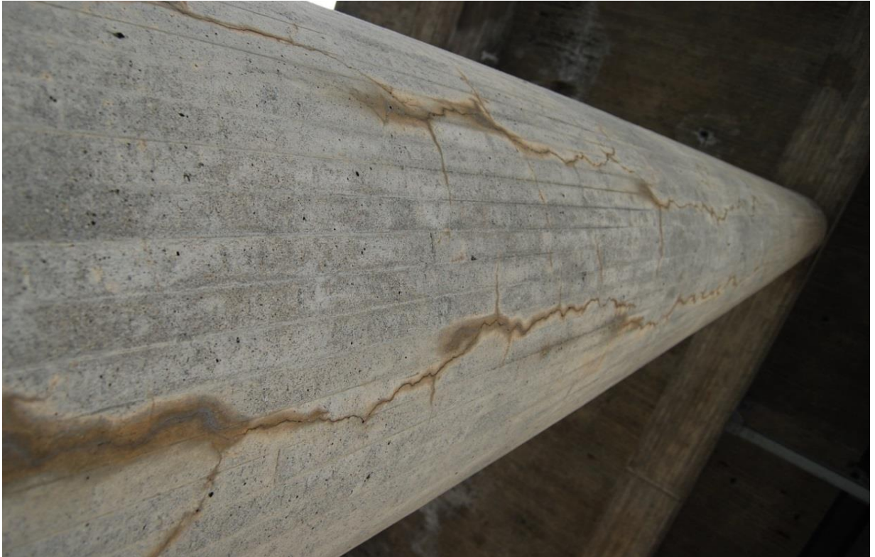
Figure 2.5. Corrosion of embedded reinforcement in column [ fot. by Maciej Wisniewski & Krzysztof Wojslaw ].
