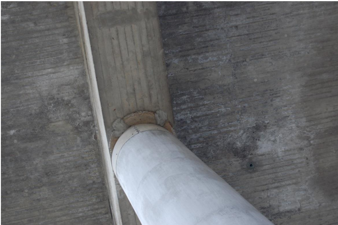
Figure 3.5 shows the upper part of column 3 in Zone 7 where the concrete has been removed. Note that not all reinforcement was welded back due to rehabilitation[56]. [ fot. by Maciej Wisniewski & Krzysztof Wojslaw ].
