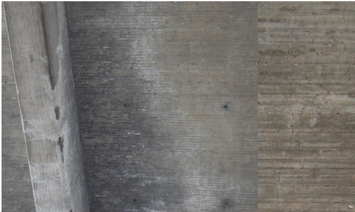
Figure 3.8 Cracks in slab in zone 1 [ fot. by Maciej Wisniewski & Krzysztof Wojslaw ].
