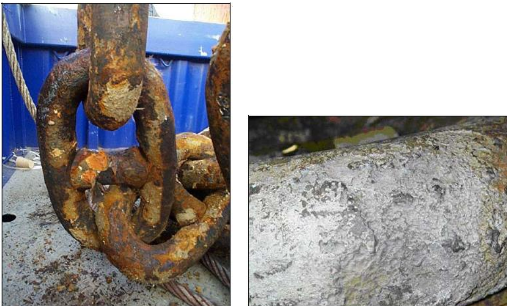
Figure 7.3: Corroded chains. The photo to the left shows general corrosion of a stud chain after 16 years' service and the photo to the right shows corrosion pitting on the curved surface of a chain link [12, p. 103-104]
