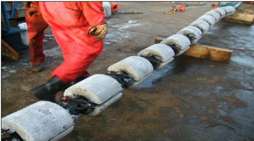
Figure 9.2: A sacrificial anode is disconnected from the cathodic protection system and brought onshore to control the rate of corrosion [12, p. 150]
