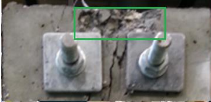
Figure 37 – Spalling of cover concrete
