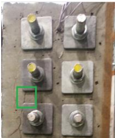
Figure 38 - First critical cracks
