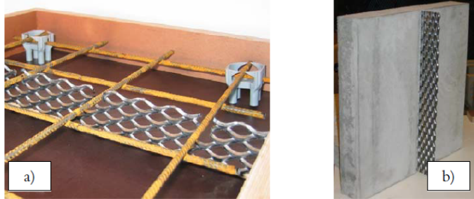
Figure 2.4: The steel mesh: (a) in the formwork, (b) prefabricated concrete slab with inserted shear connector (Lukaszewska, 2009)
