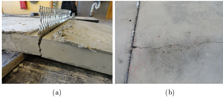
Figure 4.4: Cracking in the concrete slabs (a) right after removing formwork and (b) when mounting the slabs to the glulam
