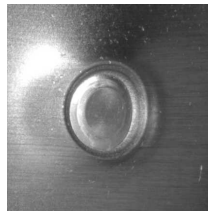
Figure 4.8: Rivet connection from C-0 test after deformation. The underside of the bottom shown.
