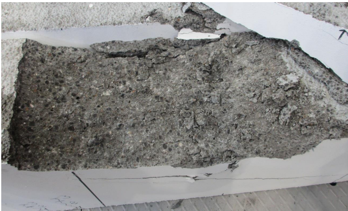
Figure 6.16. Piece of the top of beam 1B removed after testing.
