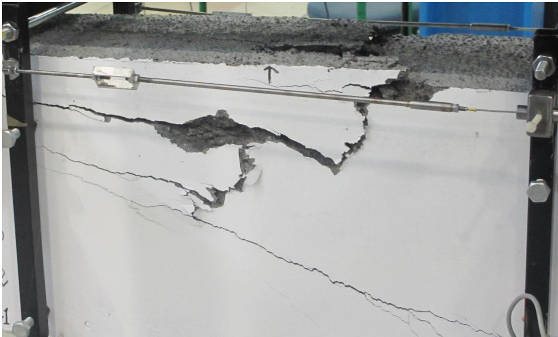
Figure 6.15. Final cracking on the west side of beam 1B.
