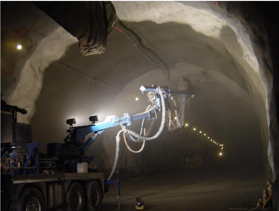
Figure 12. Construction of waterproof SCL, application of final inner layer of sprayed concrete. Test section with SCL in the Bærum rail tunnel, Norway (2009)
