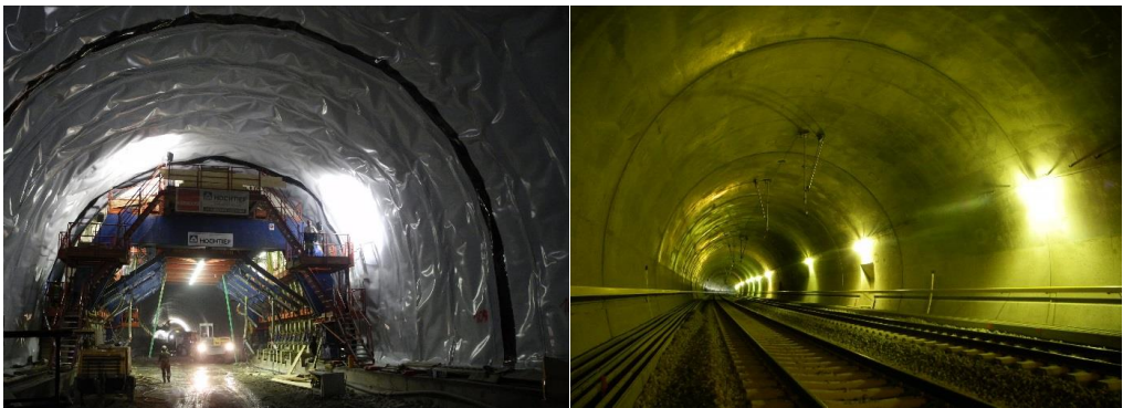
Figure 10. Photos of the cast concrete lining system during the construction of the Ulvin rail tunnel at the E6-Dovre rail line joint project, Norway, 2015. Left: installation of sheet membrane waterproofing. Right: interior of completed tunnel lining
