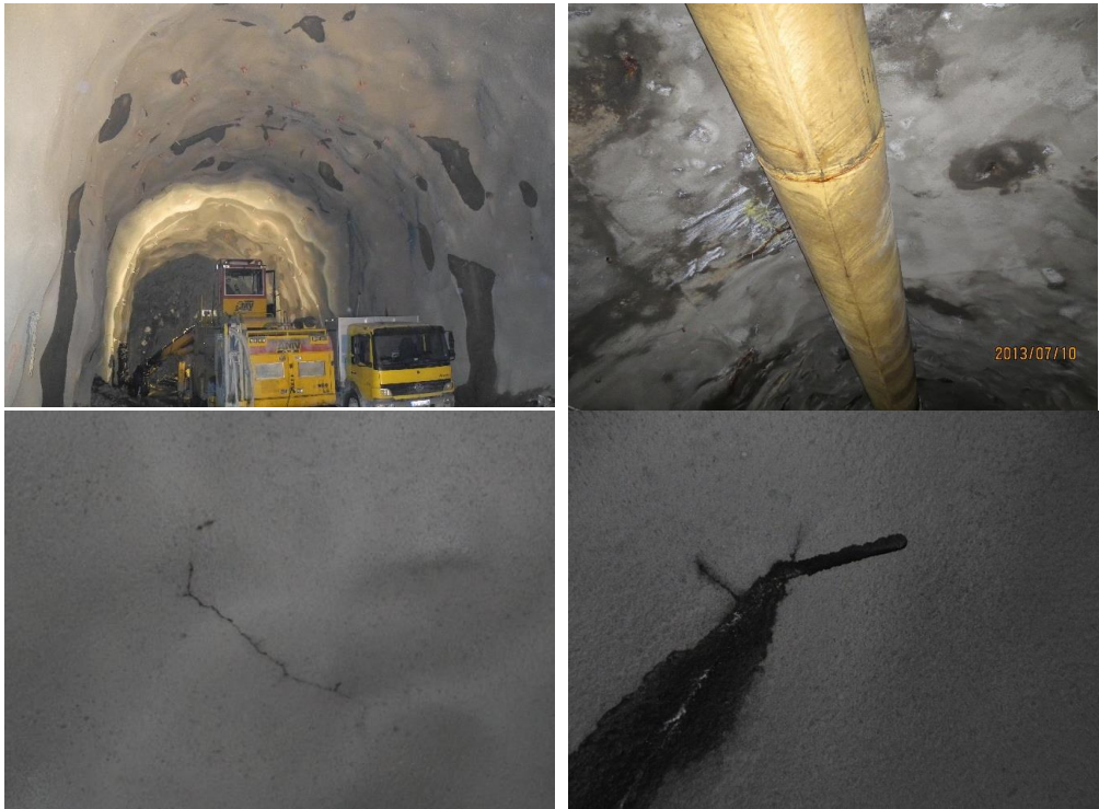
Figure 40. Constructability issues for SCL with bonded membrane experienced at test sites. Upper photos: seepage condition through the rock support lining before applying the membrane, left: Ulvin; right: Forsmark. Lower photos: typical experienced leaks through inner lining prior to any post injection works, left: Ulvin M1 damp spot in crack, right: Forsmark, leak around rock bolt
