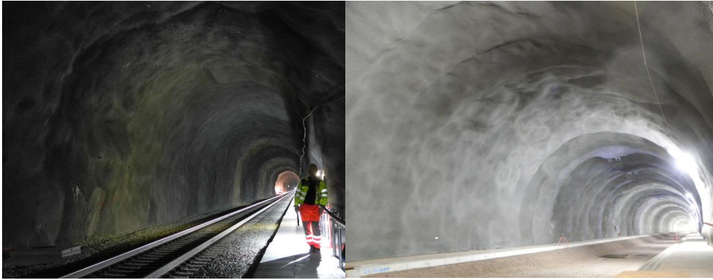
Figure 13. Photos of completed SCL with sprayed EVA based membrane. Left: The Gevingås rail tunnel, Norway (2011). Right: completed lining for a section of the twin track Holmestrand rail tunnel, Norway (2015).
