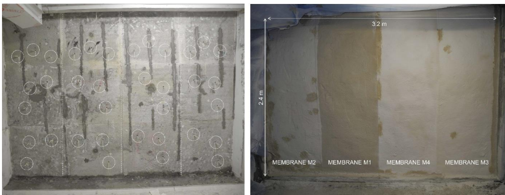
Figure 23. Photos of the freezing laboratory during the construction phase of the lining structure. Left: Rock mass surface after demolition of previous lining. The holes for water exposure are indicated. Right: Surface of lining structure with 4 different membrane products prior to the application of the inner lining of fiber reinforced sprayed concrete.
