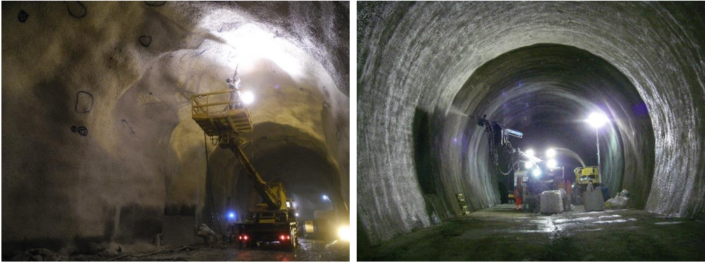
Figure 11. Construction of waterproof SCL. Left: Manual spray-application of membrane at the Ulvin test site (2011). Right: Robotic spray-application of membrane during the construction of the Hindhead motorway tunnels, UK (2009)
