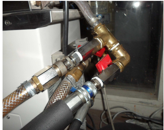
Figure 31 - Valves behind Julabo heater
