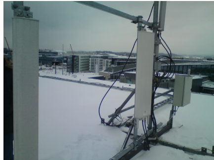
(b) Antennas mounted on the roof of the Telenor Center
