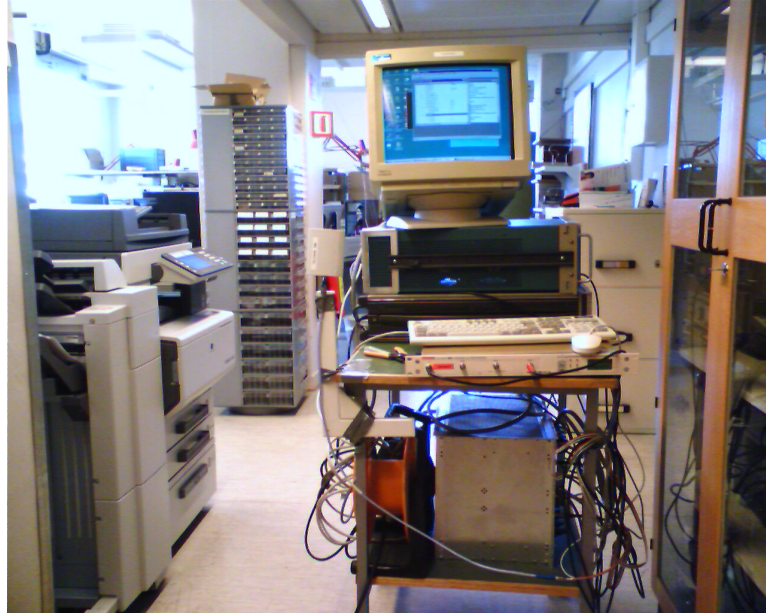
Figure B.2: Transmitter Equipment
