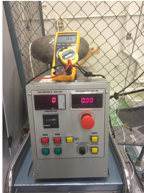
Figure 4.6: The voltage regulator (variac) that supplies the test setup with increasing voltage of a fixed rate (1kV/sec).
