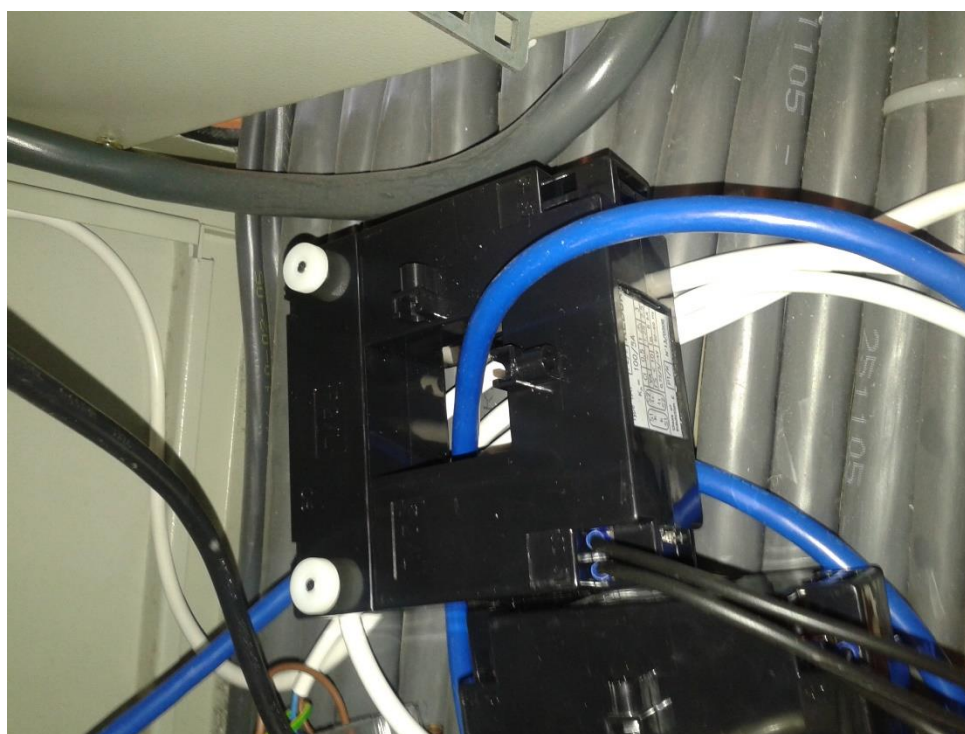
Figure 46: 100/5A current transformer. Property of SINTEF Energy Research.
