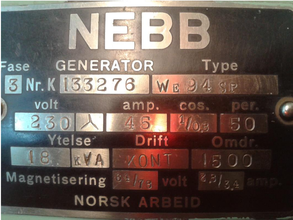
Figure A-10: The Synchronous generator identification plate. Also used as basis for the simulation model in PowerFactory as it is the only documentation that exist.
