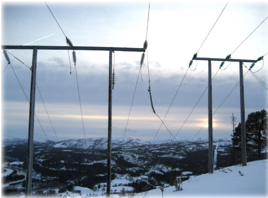
Figure 1: Photograph of the open conductor fault that caused power oscillations in NTEs network [1].
