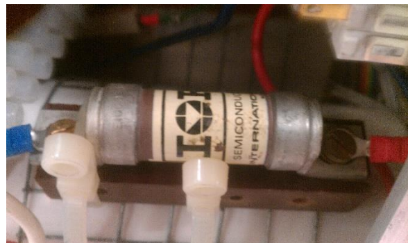
Figure 8.4.3.5: Fuse inside 3kW inverter
