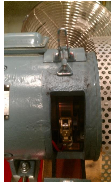
Figure 8.4.3.16: Fan set-up for preventing overheating in the DC machine
