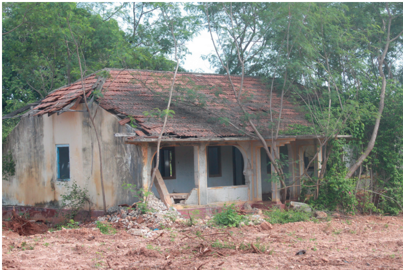
Picture 2: House left behind, damaged and overgrown by trees and plants. Jaffna, 2012
